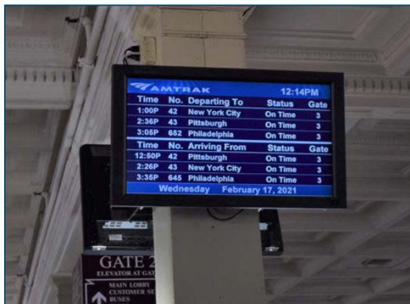
PIDS monitor at the station in Harrisburg
