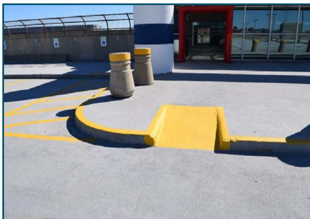
Cut out from sidewalk in parking garage at Union Station, Washington, D.C.
