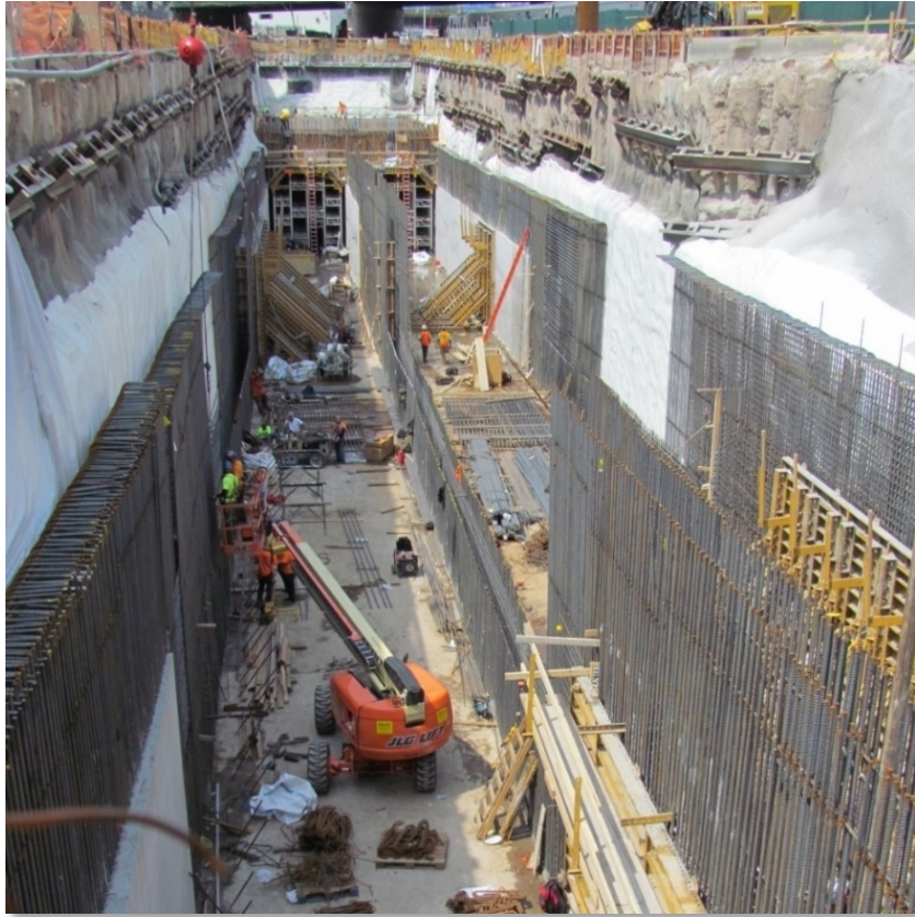
Figure 3. Construction of Concrete Casings, or “Box Tunnels,” to Preserve Right-of-Way for Hudson River Tunnels
